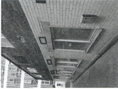
4 View of External Elevation Fitness Suite Intake and Discharge Louvers
